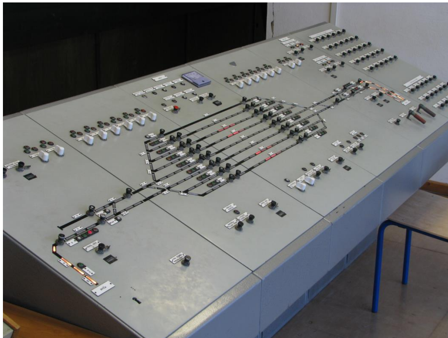
Figure 6 Control table of relay safety device type AŽD 71 with route selection method
